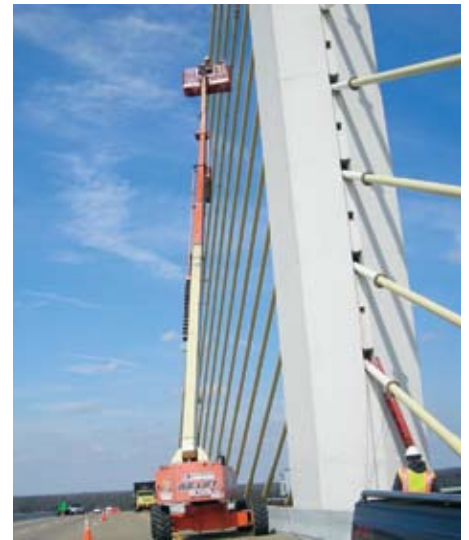
Dr. Devendra Parmar, lead principal investigator, installing acoustic emission sensors on the test cable of the bridge.
